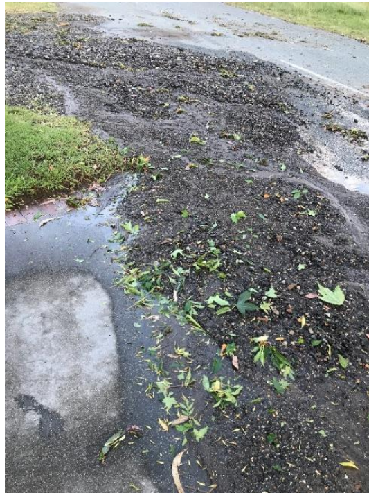
Gravel washed onto Gladstone Street, Hall
