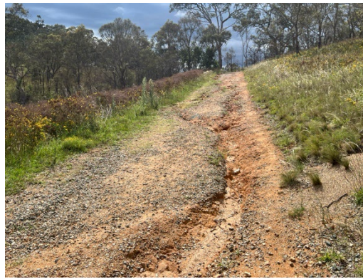
Eroded internal fire trail
