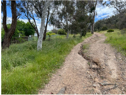
Eroded boundary fire trail
