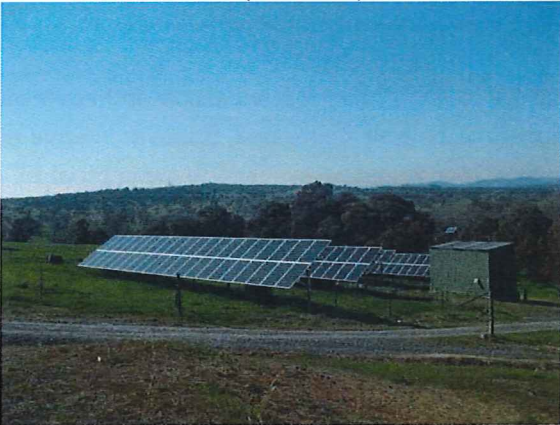
Solar Panels (Block 1582)
