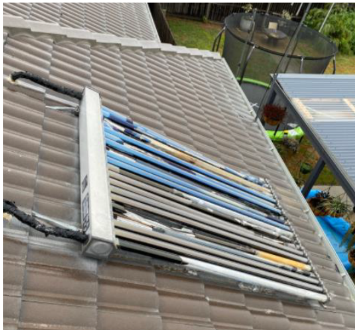
Figure 8: Evacuated tubes damaged by Canberra's January 2020 hailstorm
