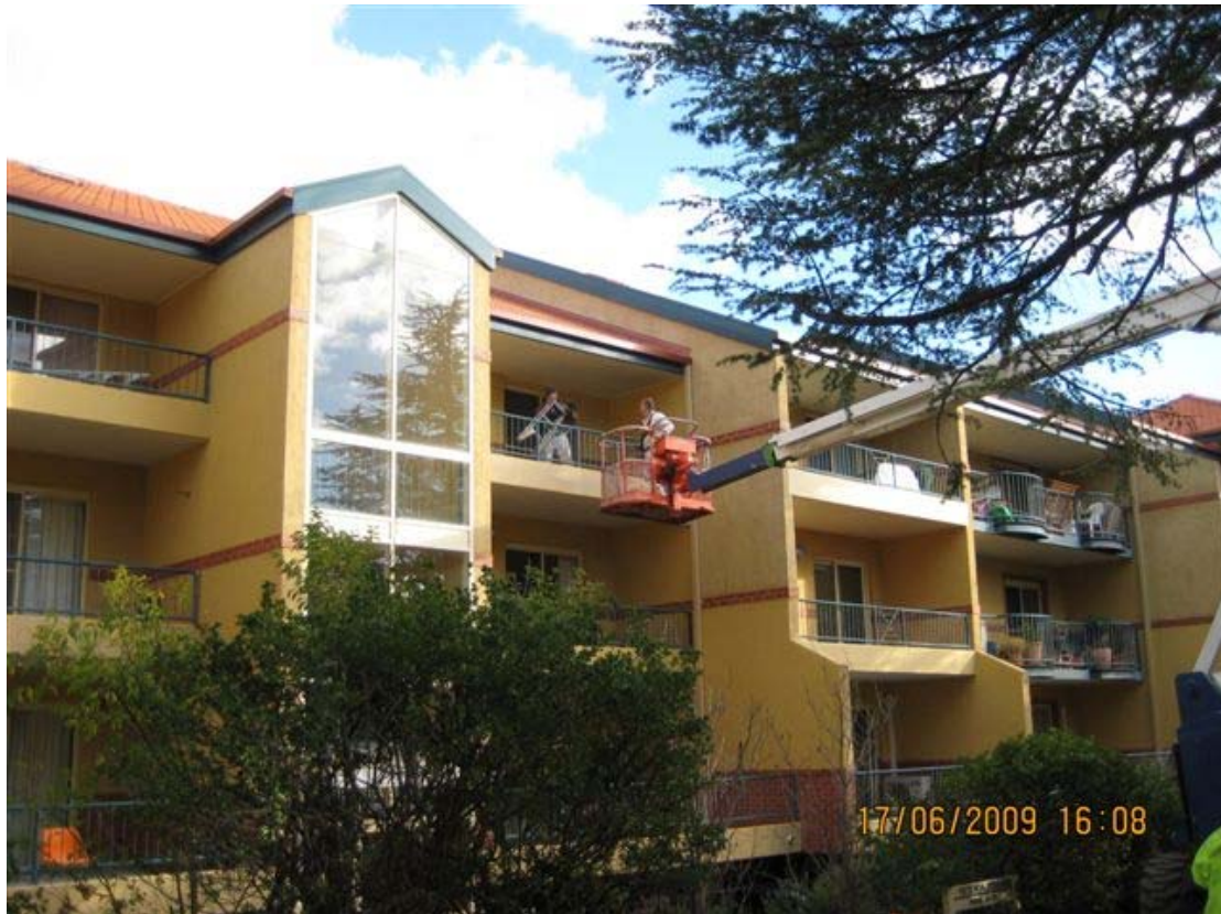
A photo of the unsafe work practice in process
