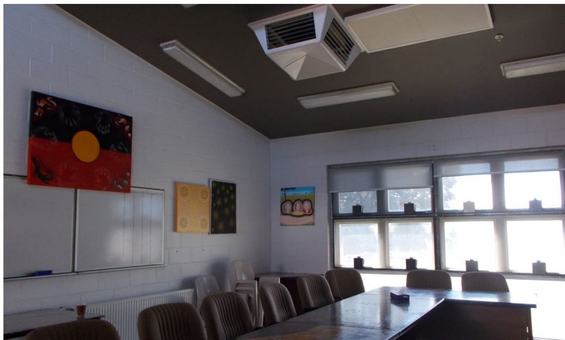
AMC Staff Administration Building – EDU Evaporative cooling
