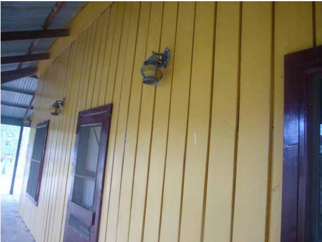
Figure 35. Shiplap timber construction of the Children's Soft Drink Building (later called the 'Spit Roast Building').
