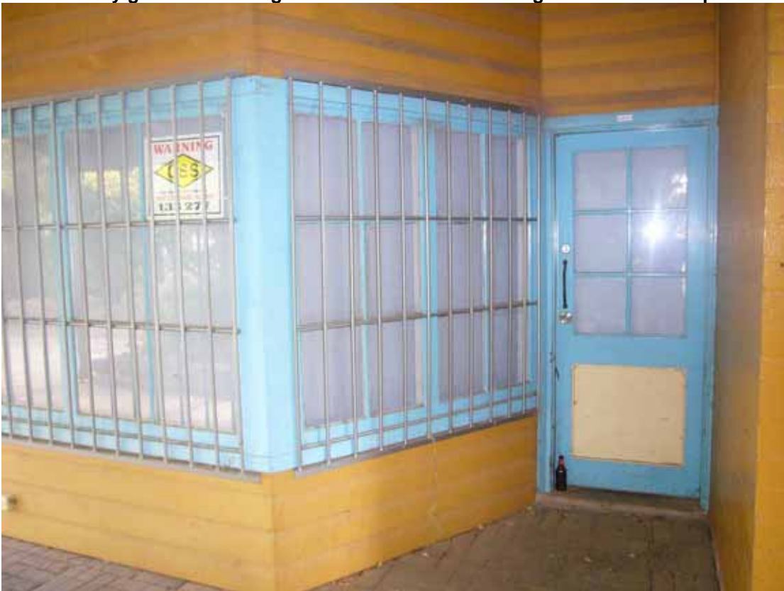
Figure 15. Close up of the front of a shop in the cottage industries building. The steel security grills are not original.
