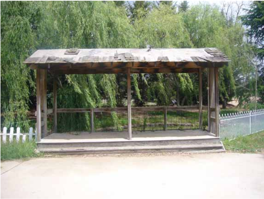
Figure 28. Covered viewing platform at catchment pond (note that the shingle roof is in disrepair).
