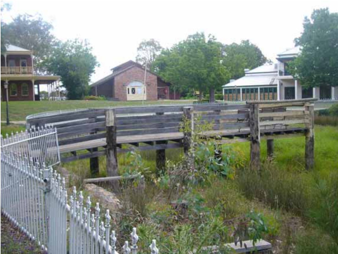
Figure 25. The jetty over the millpond (note the neglect).
