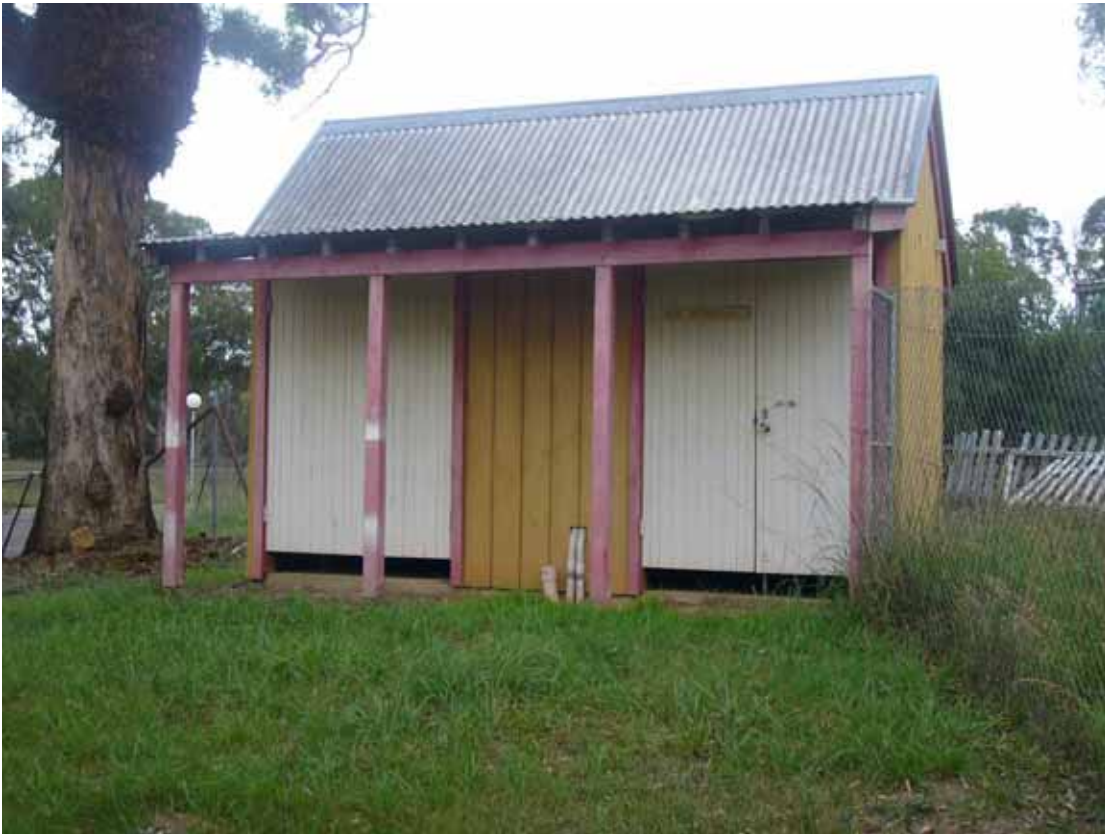
Figure 36. Switchboard building disguised as an 'outhouse' of the Children's Soft Drink Building
