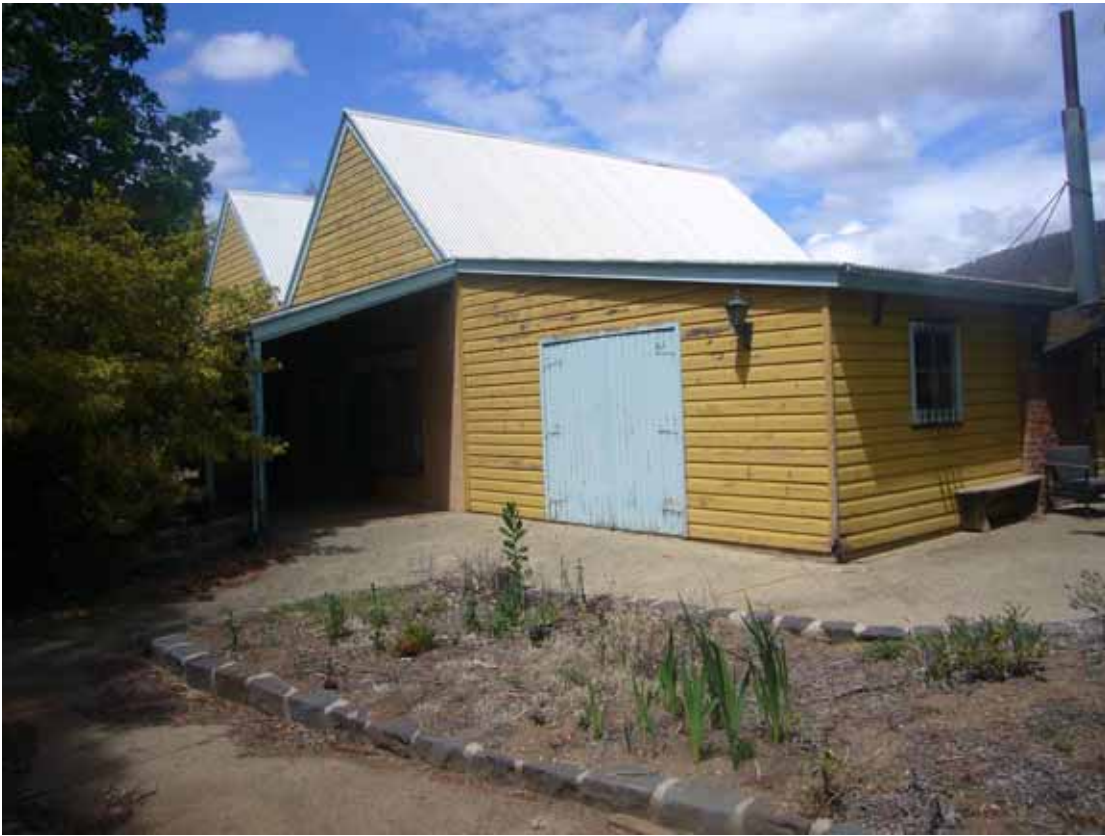
Figure 16. Front view of blacksmiths workshop (note lack of maintenance).
