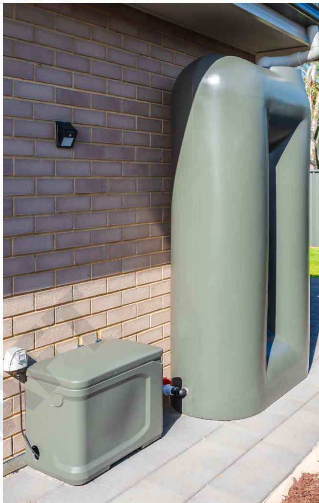
Photo 30: Rainwater harvesting systems should be designed into developments to maximise their efficiency and appearance.
