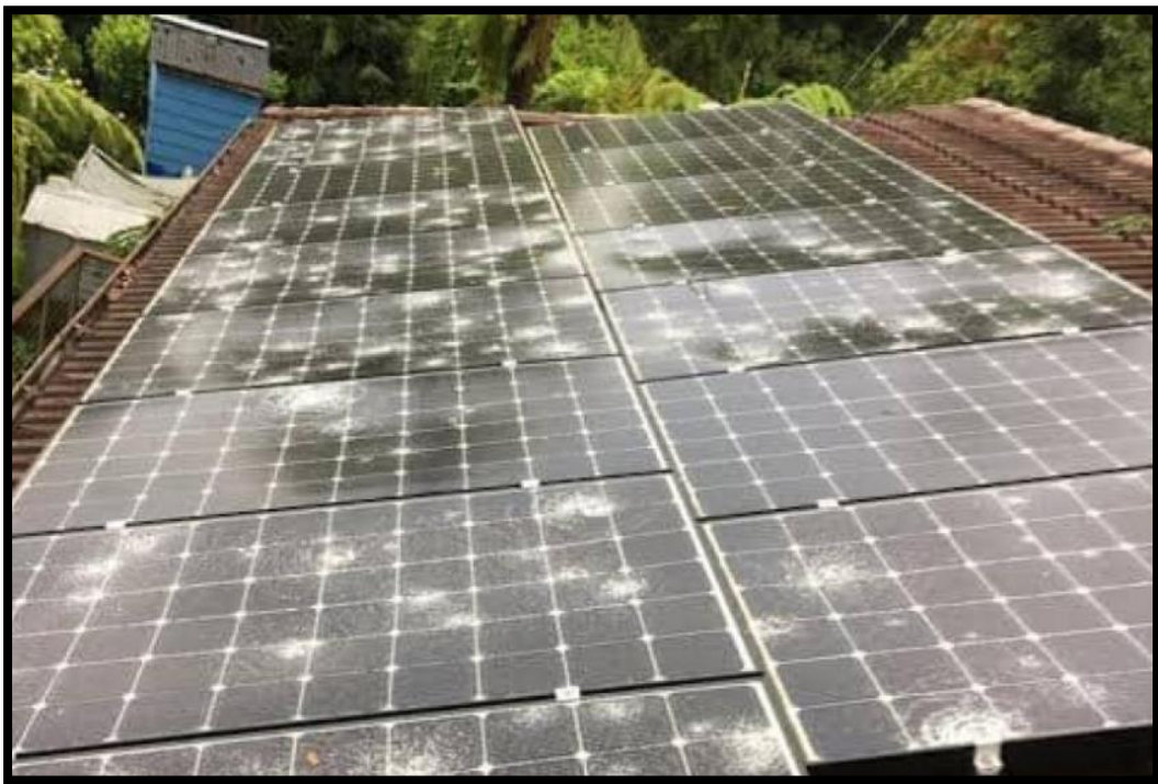
“The damage to property after the hailstorm passed over Canberra was extensive, and smashed many rooftop solar panels” (ABC News, 2020)
