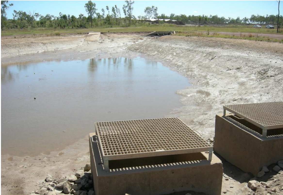
Figure 4. This basin (Bellamack NT) will ultimately be landscaped and will act as the sediment pond (pre-treatment) for a vegetated wetland. However during the subdivision construction stage it is acting as a construction-stage sediment basin while the wetland is establishing offline
