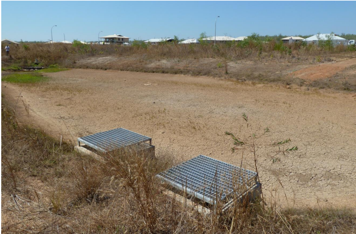
Figure 6. This basin (Johnston NT) will ultimately be a bioretention system, however until construction is complete in the upstream catchment, it has been installed as a simple sediment basin. After construction-stage sediment is removed, the drainage system and filter media will be installed and vegetation established in the system
