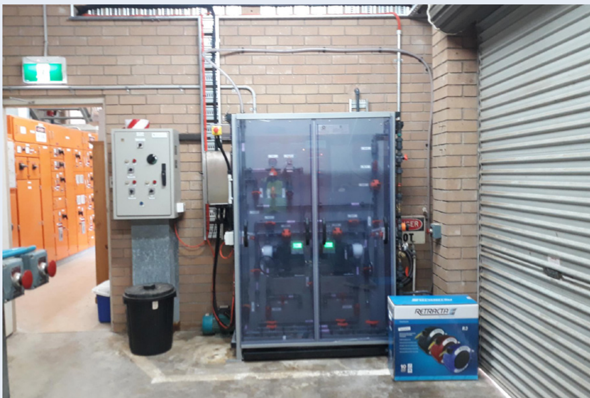
Alum dosing system installed at Yass Water Treatment Plant Photo credit: Yass Valley Council
