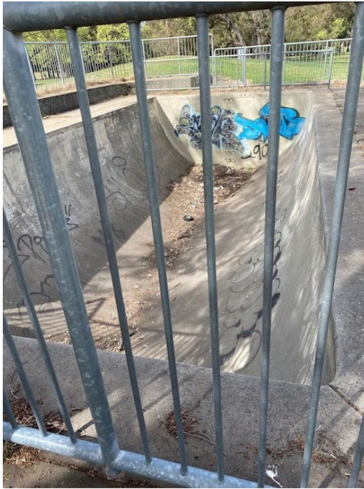
Image 6: Kambah U-Pipe. Source: Legislative Assembly of the ACT
