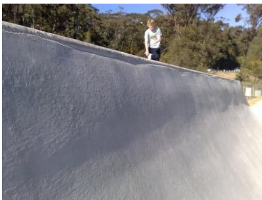
Figure 1. (Poor build quality, 2009).
