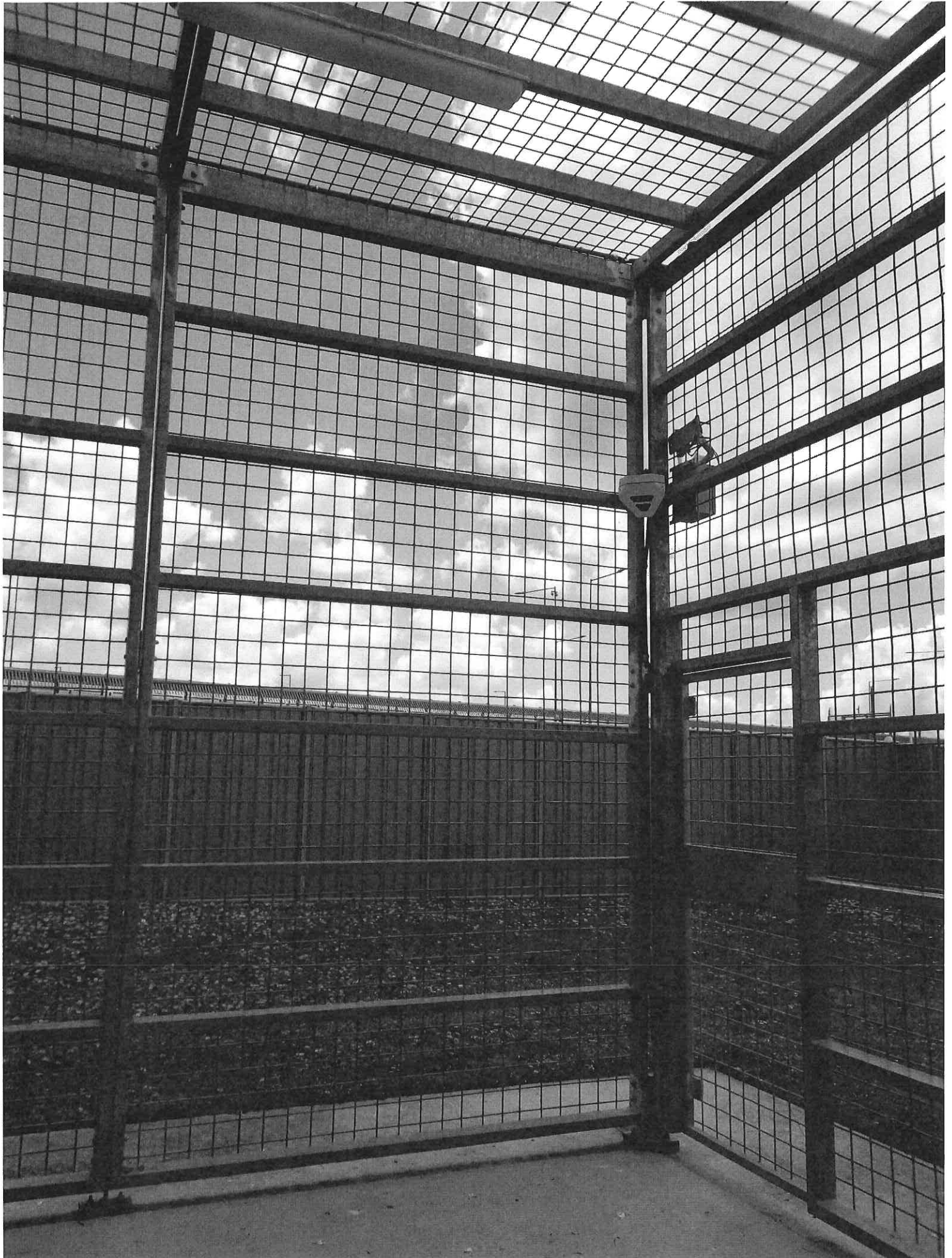
Annexure B: photographs of the general exercise yard exhibited to the affidavit of Mr Rust
