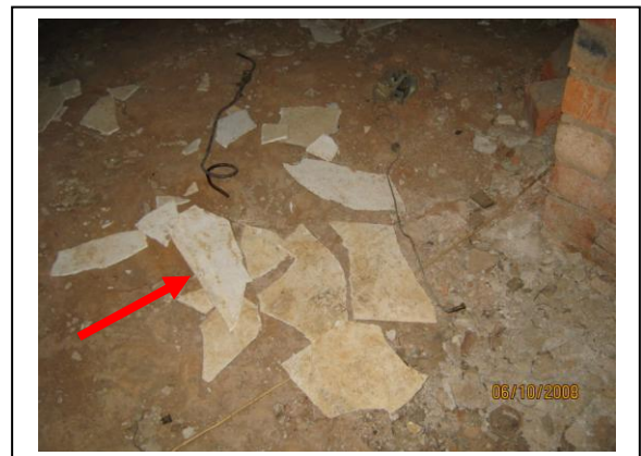
Photograph 6: Sub floor – Sheeting debris throughout (refer sample 5038 – A10)
