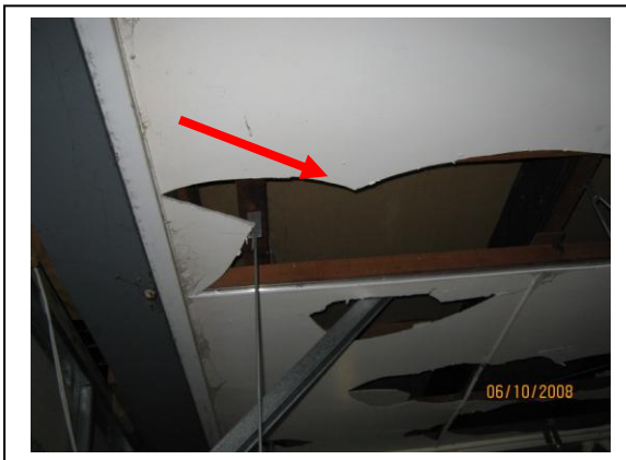
Photograph 3: Team locker area – Ceiling sheet in bulk head (Damaged) (refer sample 5038 – A5)
