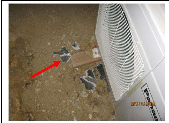
Photograph 7: Sub floor – Sheeting debris adjacent to A/C Unit (refer sample 5038 – A11)
