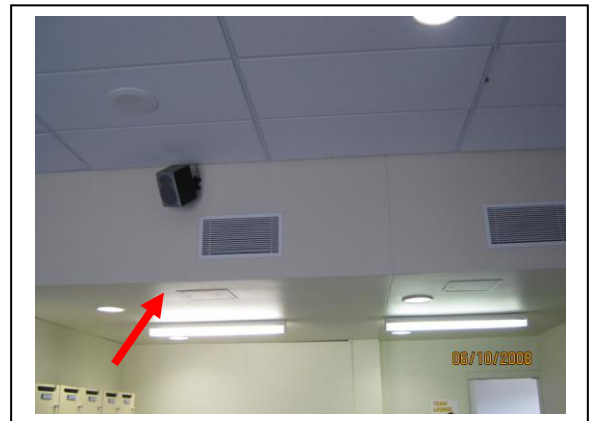
Photograph 4: Team locker area – Ceiling sheet in bulk head (Damaged) (refer sample 5038 – A5)
