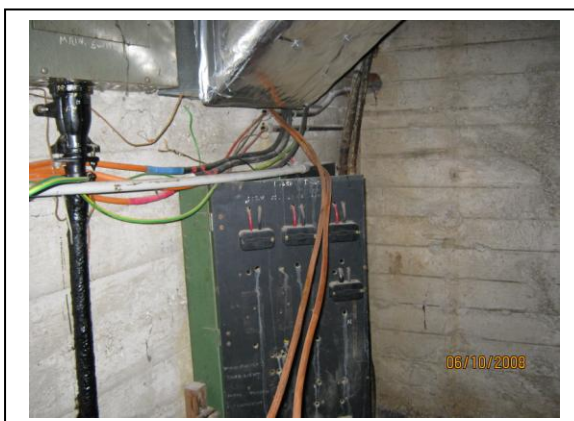
Photograph 11: Electrical switch board backing sheet – Sub floor area x4 (refer sample 5038 – VA2)
