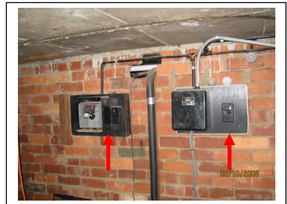
Photograph 10: Electrical switch board backing sheet – Sub floor area x4 (refer sample 5038 – VA2)
