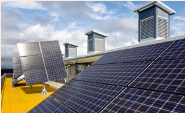
The solar photovoltaic panels on the top floor of Building K. Source Ben Wrigley
