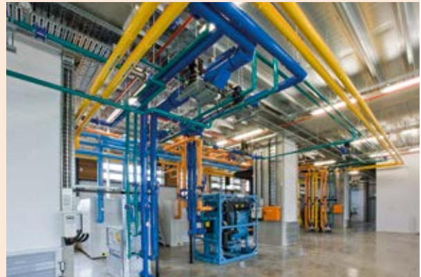
The piping network below the building which heats the building. Source Ben Wrigley
