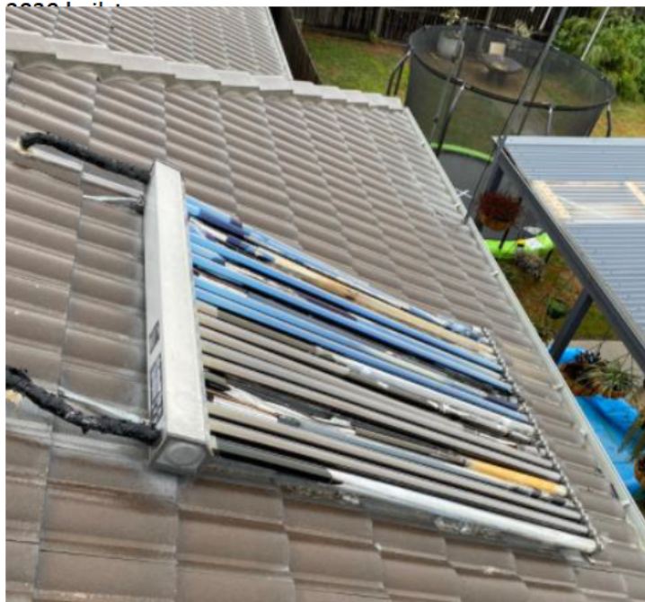
Figure 8: Evacuated tubes damaged by Canberra's January
