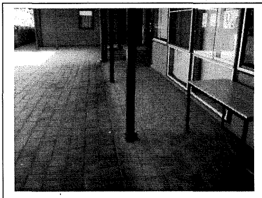
Photograph 7: Honyong courtyard verandah posts. 1 st Schedule Paint – 0.16 to 0.31% Lead Refer Sample: 5816 – P3(a,b,c)
