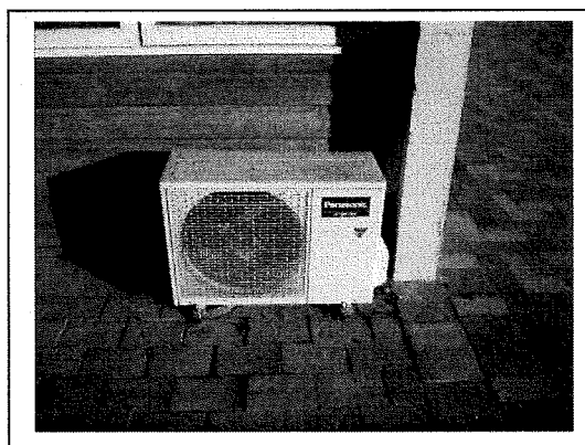
Photograph 16: Blewitt Hall Panasonic Split System Airconditioning unit – Refrigerant R410A
