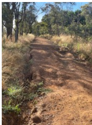
Hancock’s road erosion, Mt Ainslie January 2023
