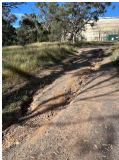
Eroded track from Rivett St to the Hackett water reservoir
